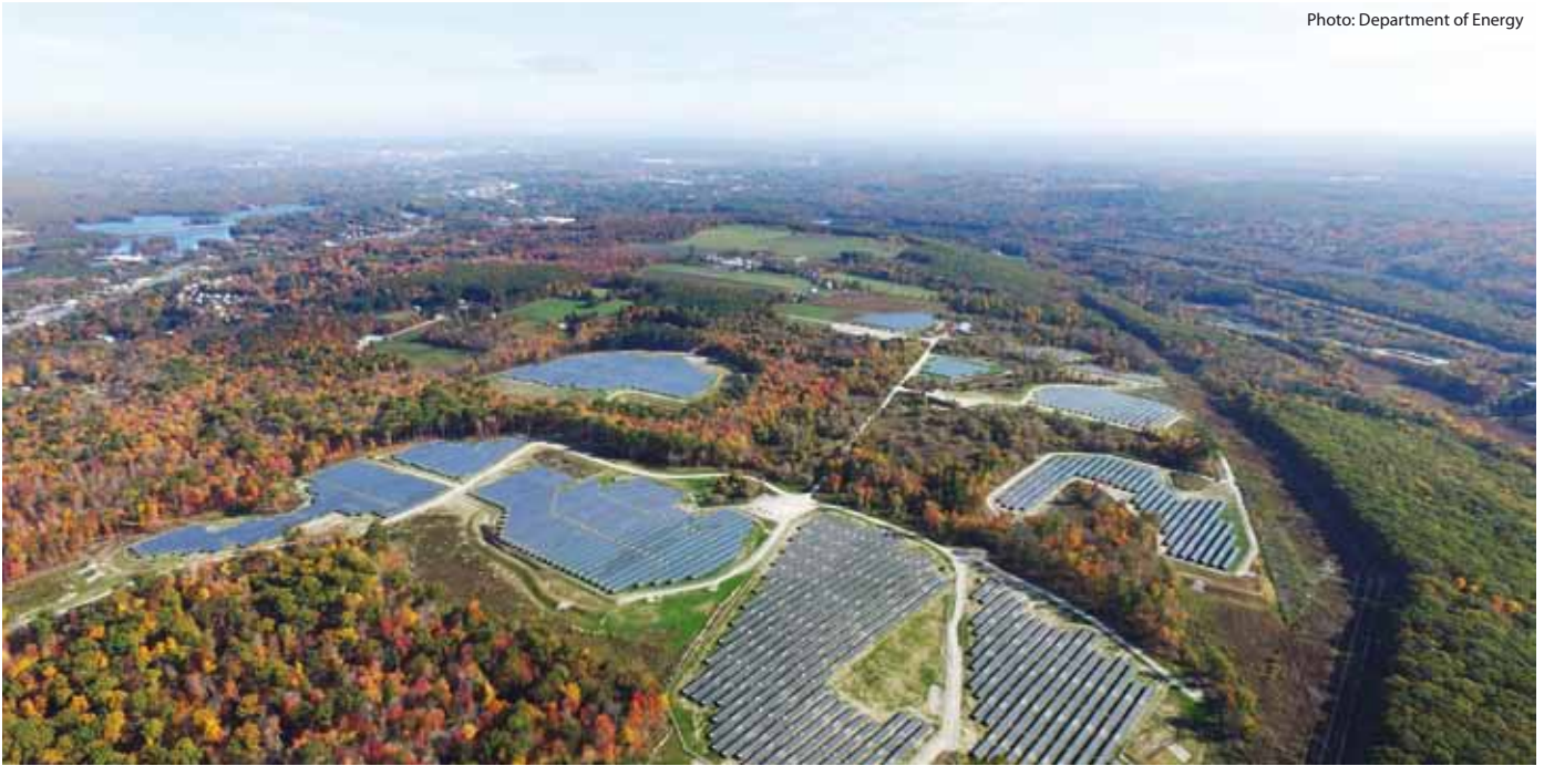
A 16.5 MW installation in Massachusetts. The state leads the ISONE region, getting 5.7% of its electricity from solar.
